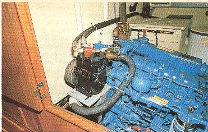
Engine mounted compressor. Silver disc at front is magnetic clutch belt-drive off crankshaft. Pipes lead to heat exchanger using engine cooling water.
