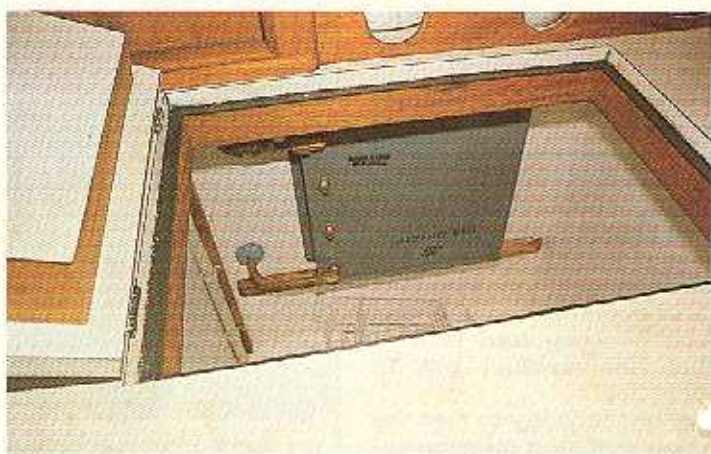
Typical hold-over plate in a fridge. Marked for 26°F it has a weaker salt solution that will freeze at a somewhat higher temperature. Note drain pickup tube in L.H. corner.
