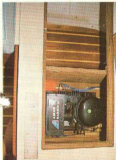
Looking down on a 12v system which cycles instead of using hold-over plates. On left is air-cooled heat exchanger; on right is hermetically sealed compressor.
